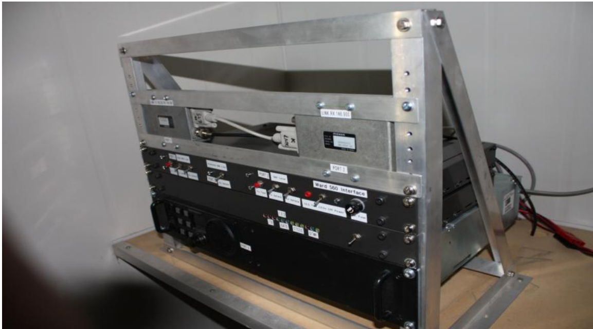
Figure 1: Linked repeater rack – starting from the top are the reverse linking radios, logic controller (all the switches), repeater controller (single switch) and finally the Yaesu VXR9000 VHF Repeater.
