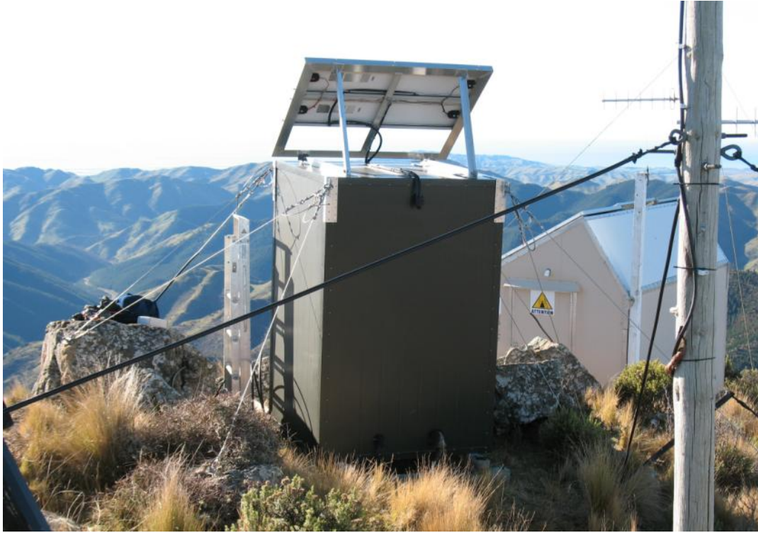
Figure 3: Blenheim 695 Repeater – a 100% solar powered site.
