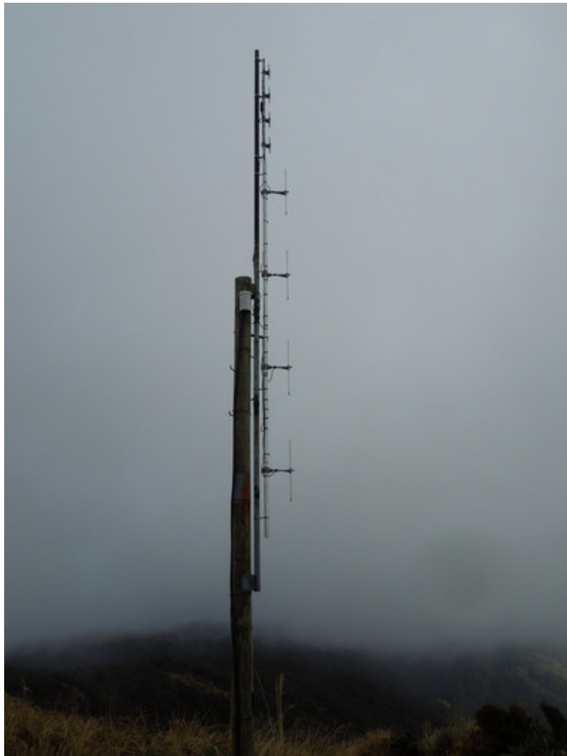
Antenna up just as the weather sets in around us
