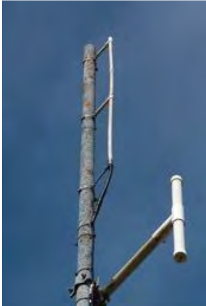
Figure 7: The installed collinear on the antenna pole at Mt. Climie. The larger antenna below the collinear is the top dipole of the VHF Stacked array for Climie 5425, data/voice repeater.
