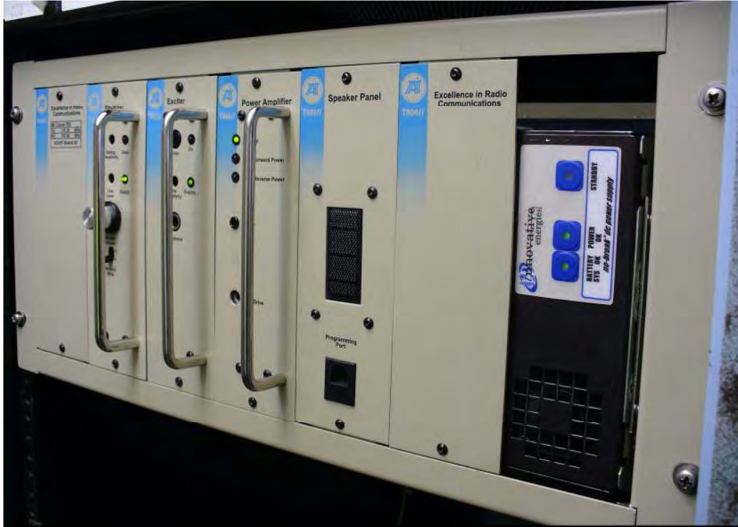
SR250C fitted to T800 VHF repeater 147.300 MHz.
